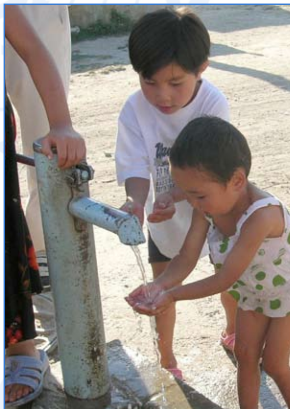
Figure 8. New water supply system in a village of Issyk-Kul oblast Source: V. Djudemisheva
