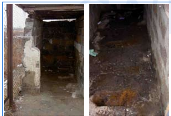
Figure 2: Exterior and interior of a latrine for 360 pupils: no privacy, unhygienic, cold and slippery during wintertime Source: WECF
