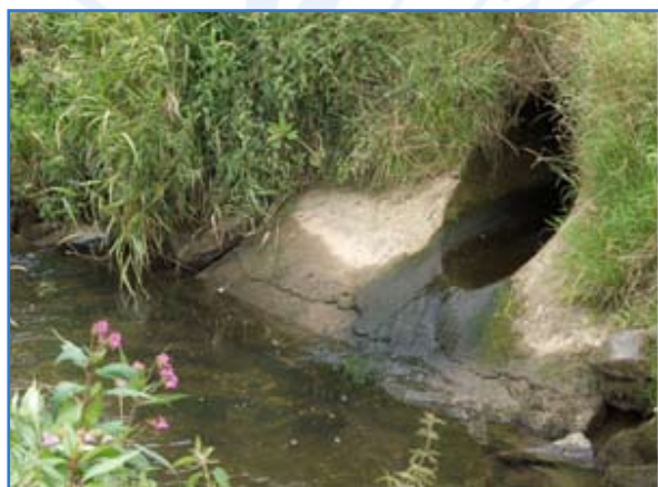
Figure 1: Discharge of treated sewage leaving the STP
