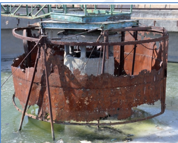
Figure 5: Central WWTP in Darkhan
